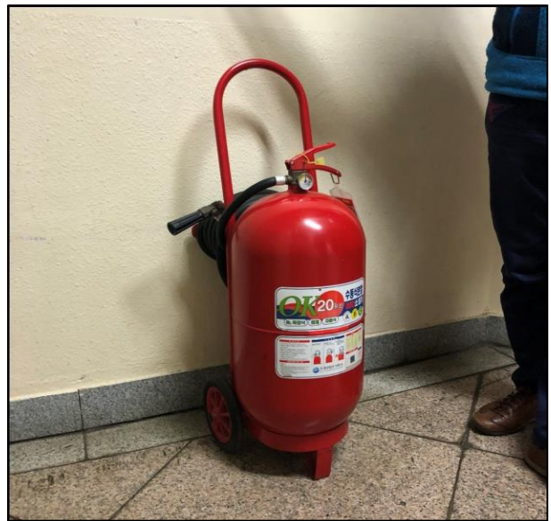
Big Fire extinguisher near gas plant room
