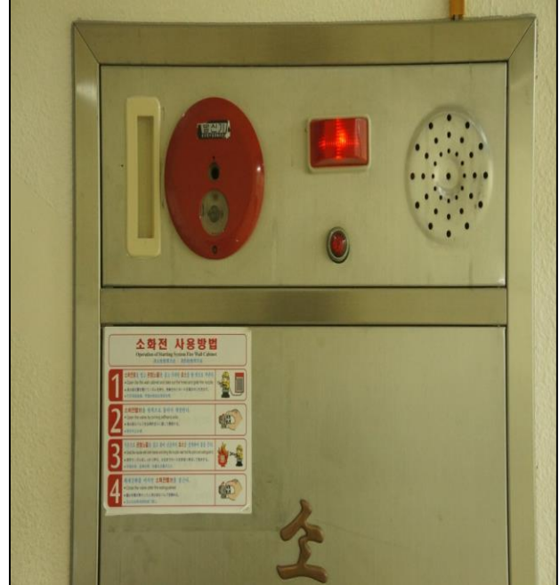
Fire wall cabinet with instruction to use
