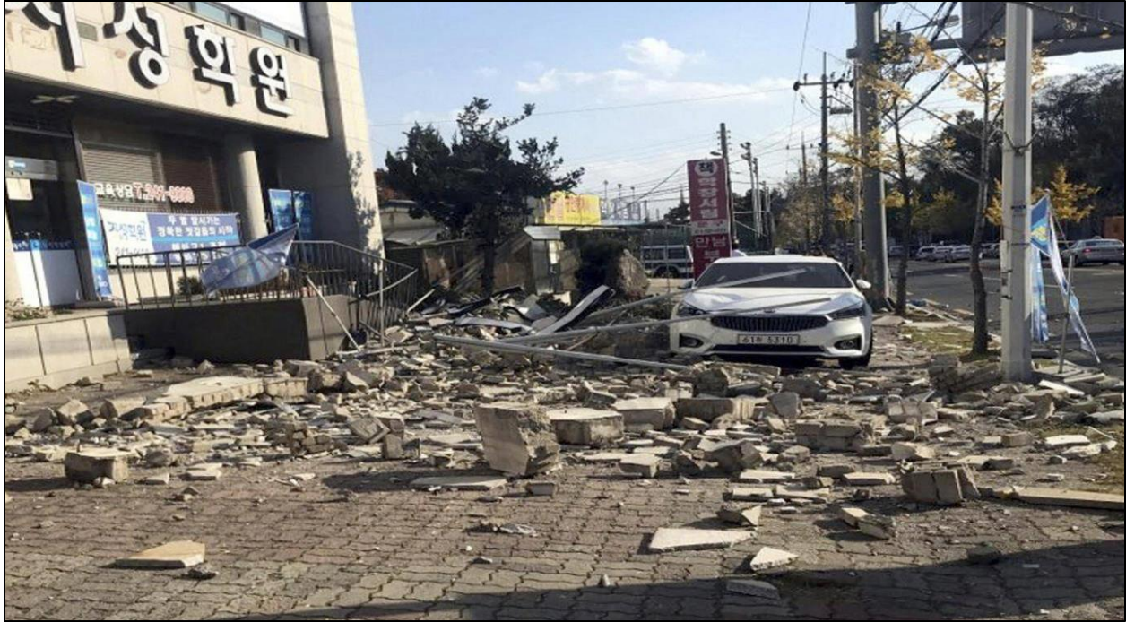
The earthquakes rattled Handong Global University campus in Pohang, destroying walls of one of the campus buildings
