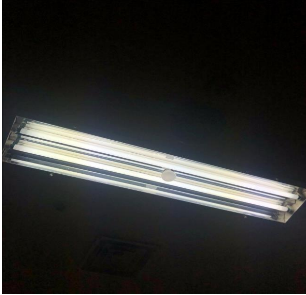
Emergency lights will keep lighting for one hour in case of shut down.
