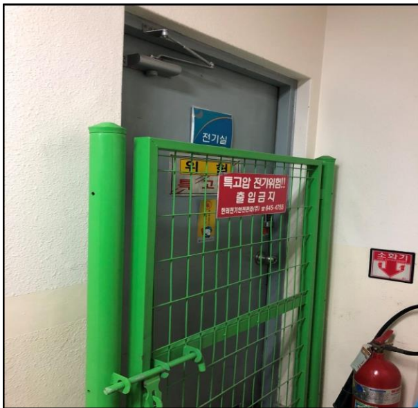
Gas plant room with extra door to avoid misshaping
